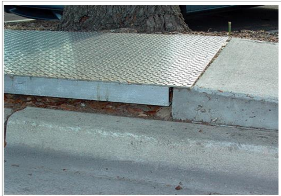
Figure G7. Sidewalk bridging over tree roots. Photo: Edward F. Gilman, Professor, Environmental Horticulture Department, IFAS, University of Florida
